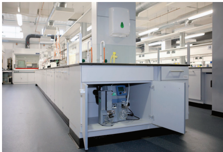
One pump - many users: network installation with Peltronic cooling without water connection for solvent recovery
