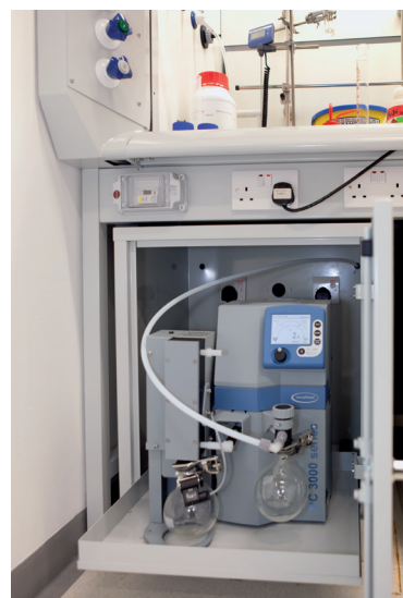
Chemical network pumping unit under the exhaust hood, with solvent recovery
