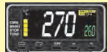
Example of over-temperature limiter
